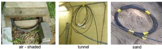
Fig. 2 Illustration of the ambient temperature measurement at various installations
