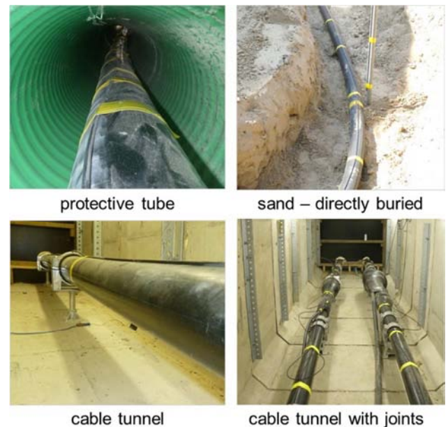
Fig. 1 Four installations at which the RTTR system was tested
